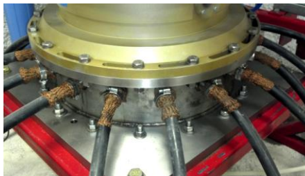
Figure 3.12—Twelve parallel high voltage output cables at the base of the PFL structure
