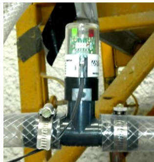
Figure 3.13—Water conductivity meter
