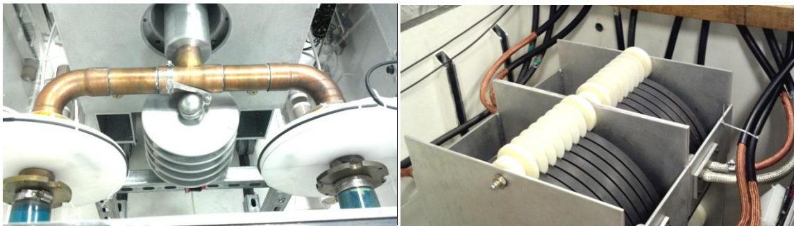
Figure 7.10—Inductive voltage adder output connected to parallel water resistor load (left), high voltage cables connecting to inductive voltage adder (right)
